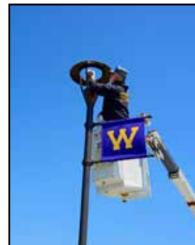
Inspecting LED lights
