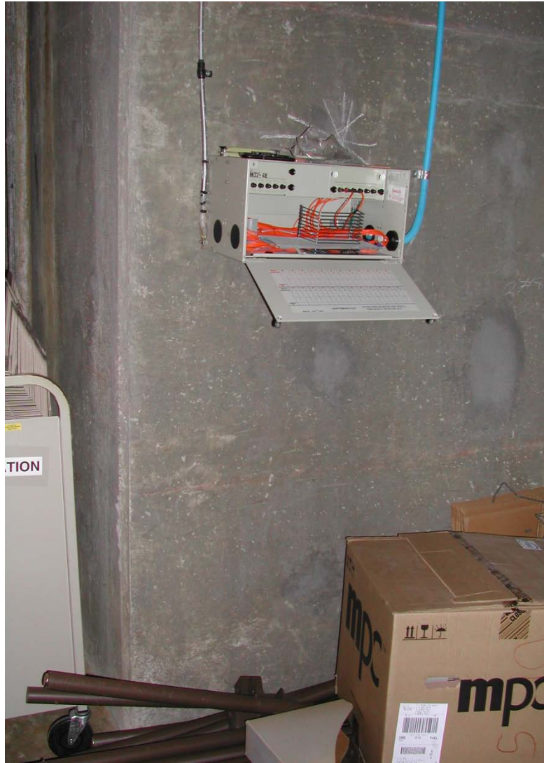
Library fiber entrance
